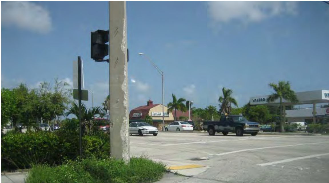
Damaged Signal Pole at northeast quadrant of Hallandale Beach Boulevard and SW 40 th Avenue
