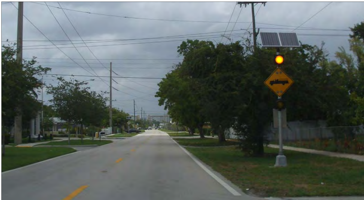
Fire Station Warning Beacon (SW 40 th Avenue)
